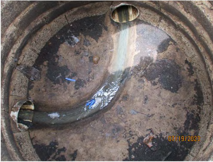
Photo #: 28 Taken by: Joshua Grosvenor Entity: Neosho WWTP Permit: MO0104906 Location: S Neosho Boulevard and W South Street Description: Manhole with the greatest frequency of overflows, during high flow events. Date Taken: July 19, 2023 Media: WPCB
