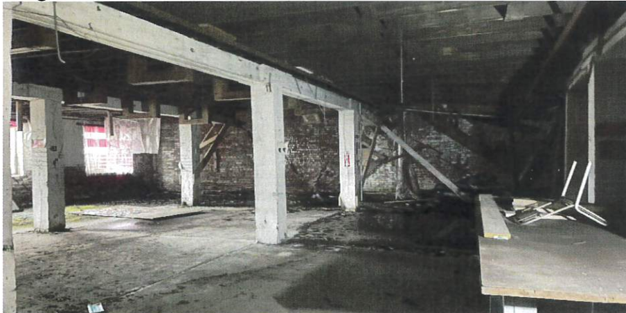
Image 2- Second story collapsing
