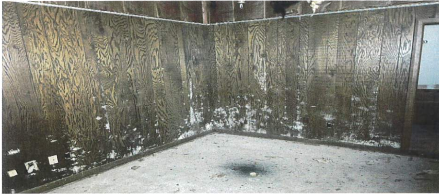
Image 1- Visible mold on interior walls
