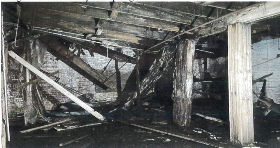
Image 3- Second story collapsing
