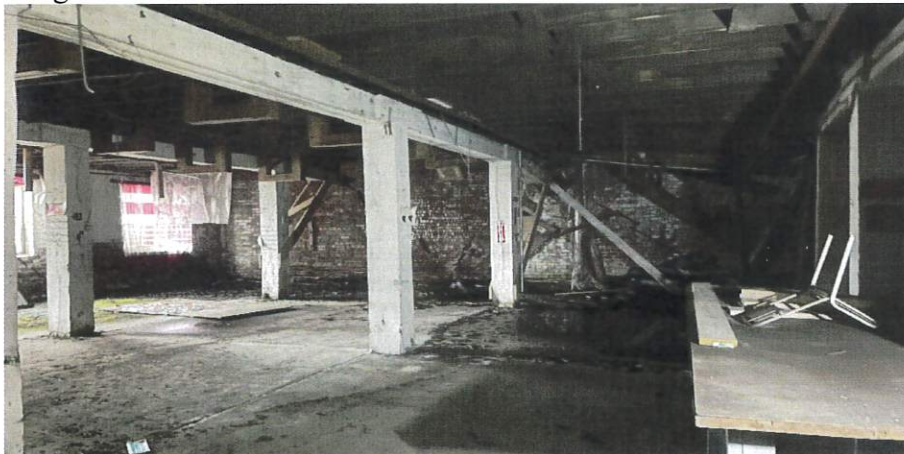
Image 2- Second story collapsing
