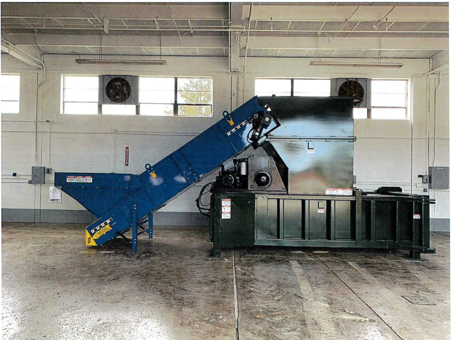
WEST VIRGINIA ARMY NATIONAL GUARD 2021 THB-6048 INSTALLATION
